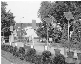
Fig.6 Solar Street Lighting
