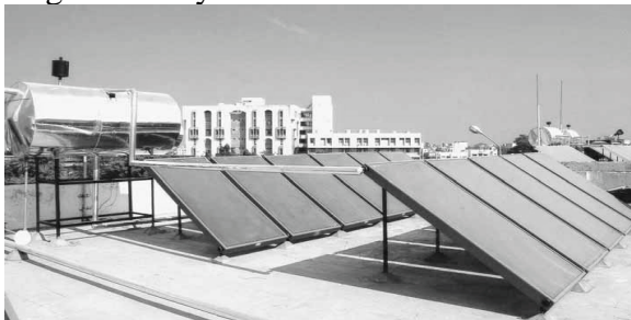
Figure 5. 3,000 LPD Solar Water Heating System installed at a Govt. Medical College Hostel in Bhavnagar, Gujarat,
